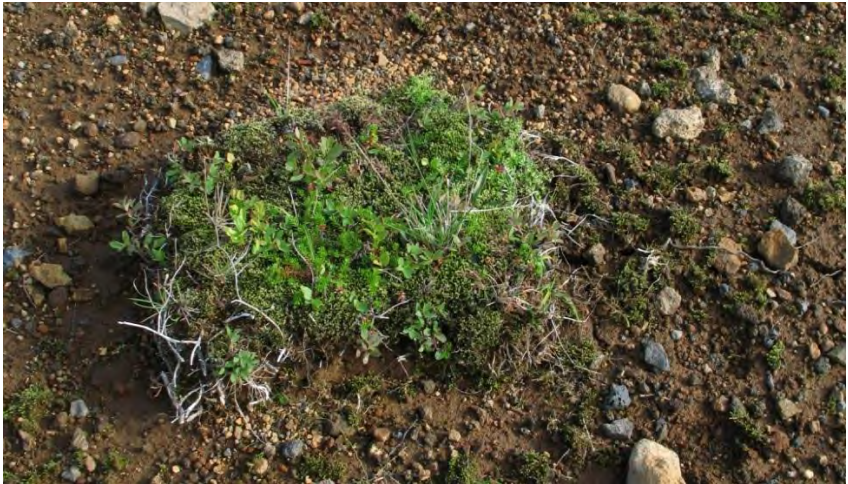
Transplanted turf used to restore natural vegetation after construction work in Hellisheiði, Iceland. Photo: Ása L. Aradóttir.
