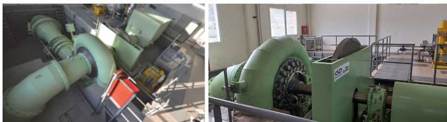
Fig. 49 The Ilarion Small HPP (SHPP)
