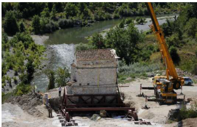
Fig. 50 Relocation of the church of Panagia Tornikiou to a higher ground
