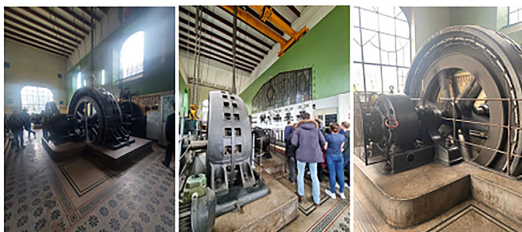
Fig. 32 Powerhouse and hydropower units installed at Timișoara SHPP
